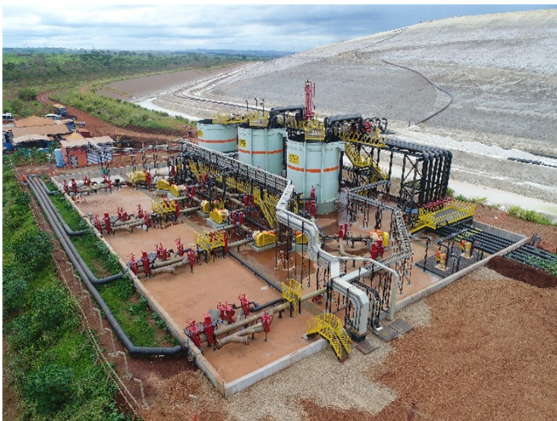
Figure 1: U-640 Gypsum Pumping Unit (Mosaic Fertilizantes)
