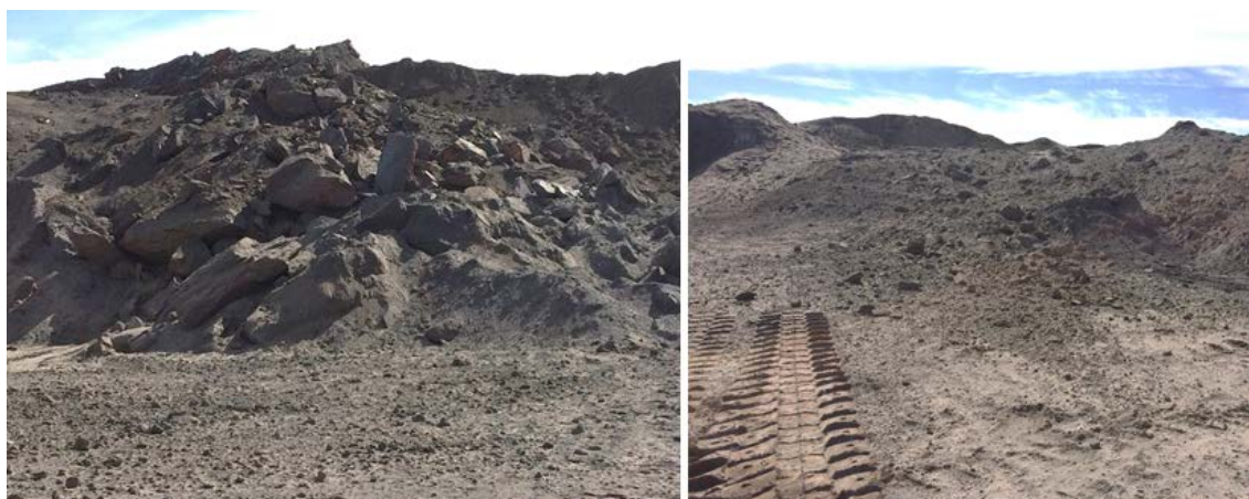
Figure 9 – Muckpiles from conventional blasting (left) and blasting based on geophysical/geological model (right).
