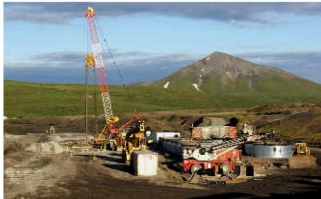
Figure11 - Cut-off wall installation with trench cutter BC 40 at Red Dog mine, Alaska
