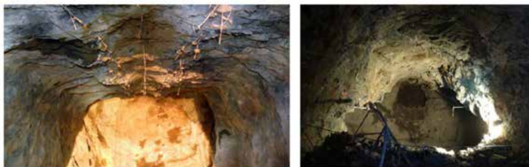
Figure 8: Photograph of TS_N195_E4 (left) and TS_N157_E4 (right), showing the destruction of cable-bolts and the preservation of the silhouette of the gallery respectively (both photographs are courtesy of the Engineering Department of Orosur Mining Inc.)
