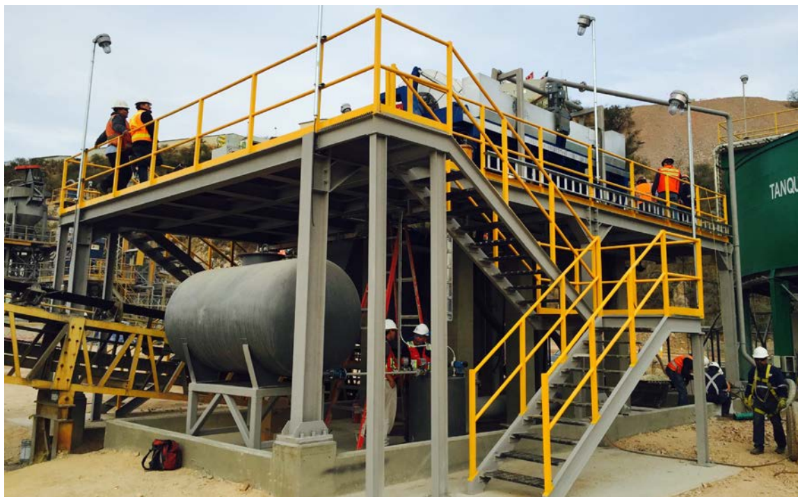
Figure 6 – Ceramic Disc Vacuum Tailings Filtration Plant, Completed (December 2015)
